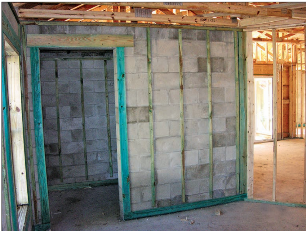
Figure 3-4: In-home safe room under construction; the CMU walls of the safe room are fully grouted and vertically reinforced with steel reinforcing bars from the foundation to the concrete roof deck (New Smyrna Beach, FL, 2007)
